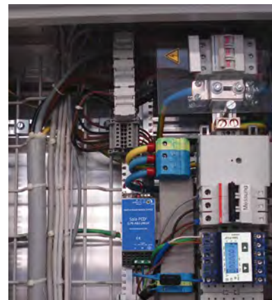
▲ Built-in current converter directly in the cable duct
