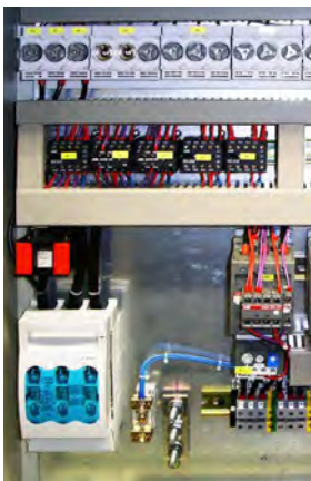
▲ Current converter in switch cabinet
