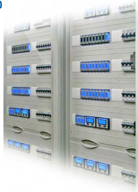
Many energy meters in the smallest space ►
