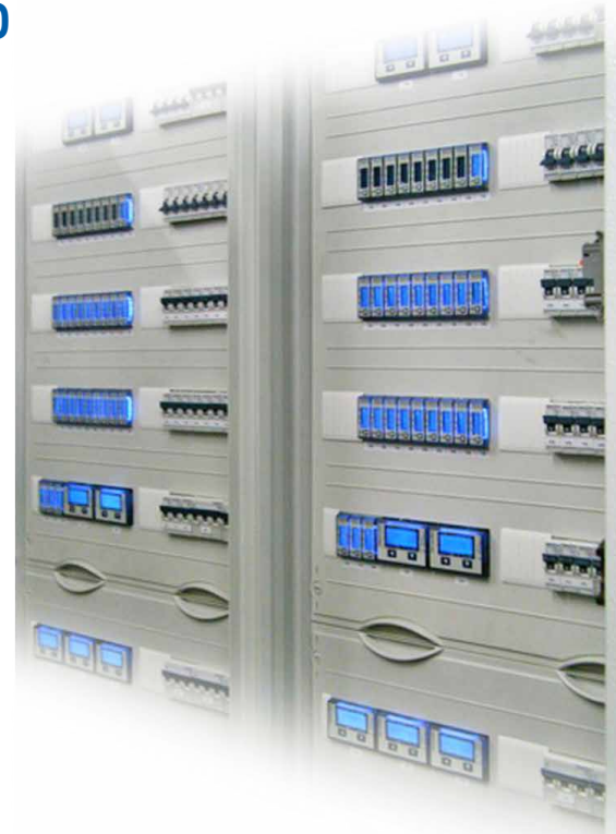
Many energy meters in the smallest space ►
