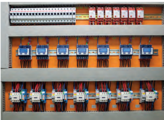
▲ Measuring consumption of heating
