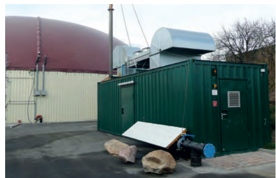
▲ Biogas plant Cavertitz – view of the combined heat & power plant container with 500 KW installed power; Fermenter in the background
