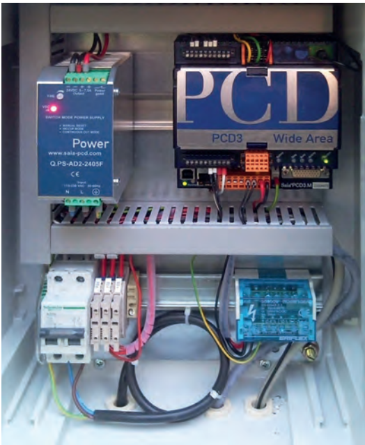
▲ Cabinet in remote site (pumping station)
