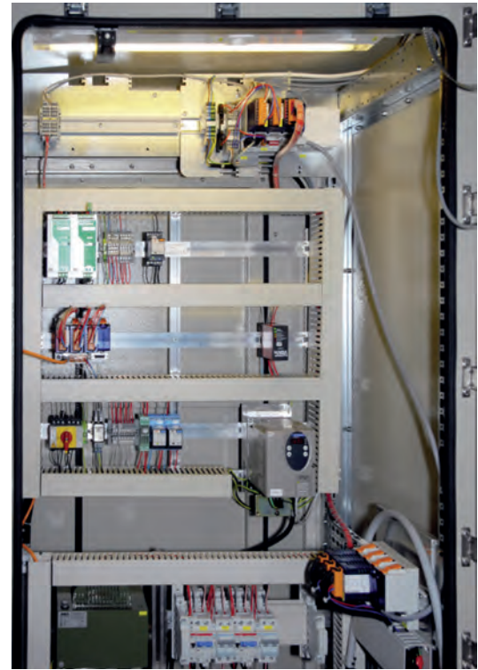
▲ Cabinet after conversion
