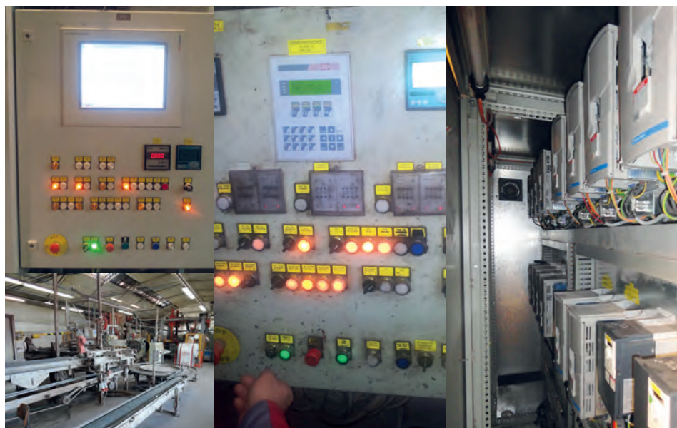
◀ New operator cabinet, Productionline, Old operator cabinet, Powersection
