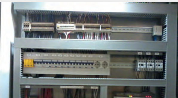
▲ Inside new panel in technical room
