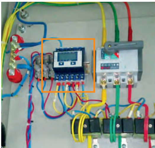
▲ Energy measurement for distributed electrical cabinet and major M&E equipment
