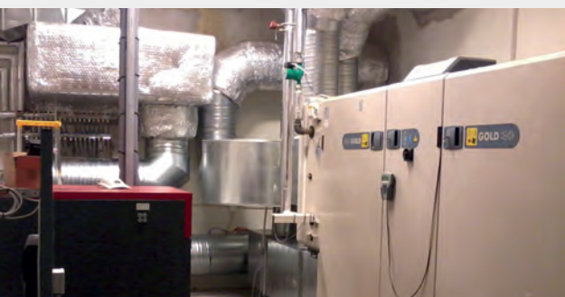
▲ Communication with Swegon HVAC Modbus
