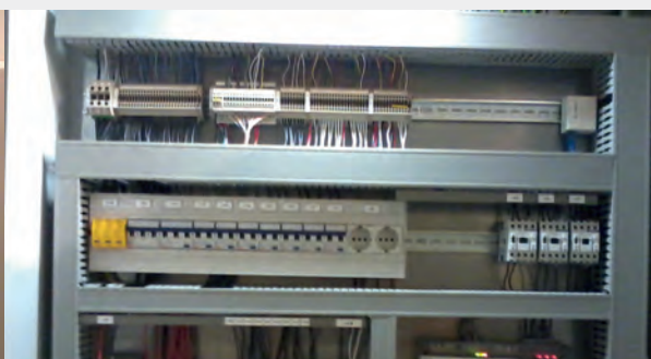
▲ Inside new panel in technical room
