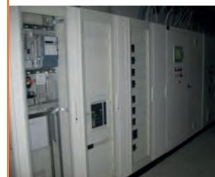
▲ Distribution cabinet + MCR
