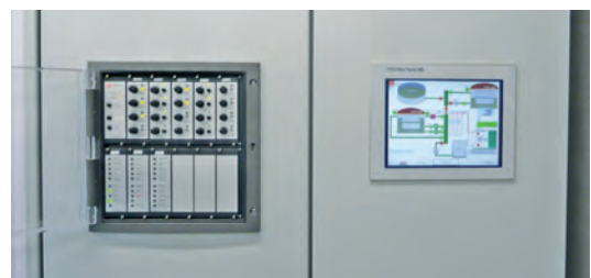
▲ Operator interface with manual emergency operation and 10 inches Saia Burgess Controls Web Panel form the basis for a comprehensive and safe operation of the plant on site
