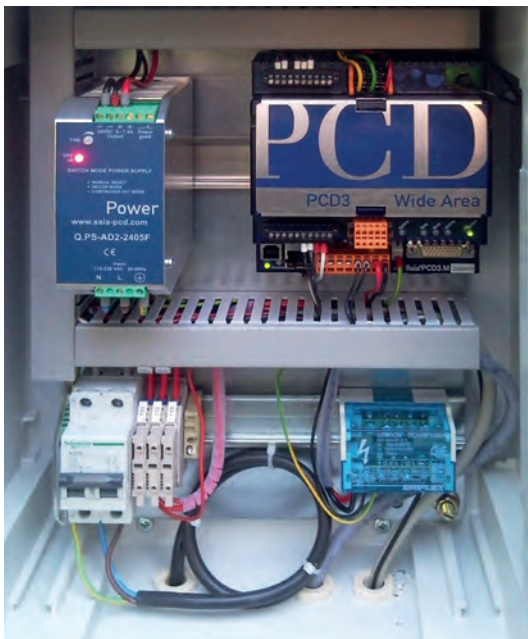
▲ Cabinet in remote site (pumping station)
