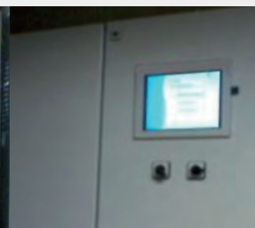
▲ New panel in heating central
