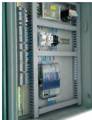
▲ Network type controllers for entire project and major M&E equipment
