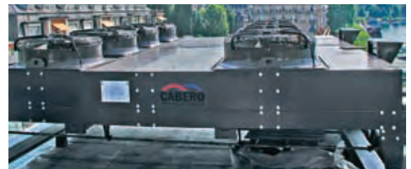
Colour-coordinated recooling unit on roof
