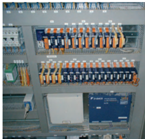
Switch cabinet with Saia®PCD3 BACnet® station (top left) and Daikin's D-BACS gateway (bottom right)
