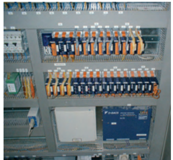
Switch cabinet with Saia®PCD3 BACnet® station (top left) and Daikin's D-BACS gateway (bottom right)
