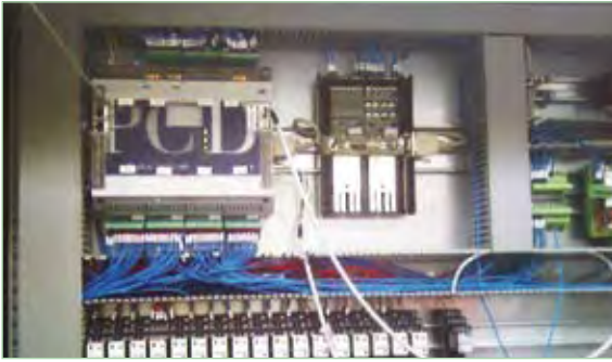
View into the cabinet of the new machine: Saia®PCD2.M5540 with Profibus connection.
