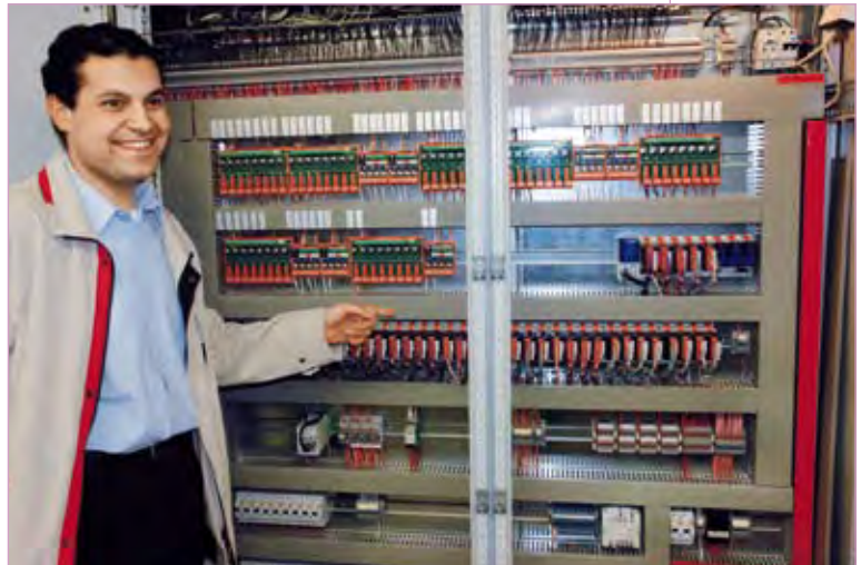
The customer's smiling Project Manager in front of a control cabinet with some Saia®PCD3.M5 controllers.
