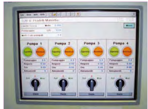
Web control masks for pumping station on a Saia®PCD Web-Panel CE
