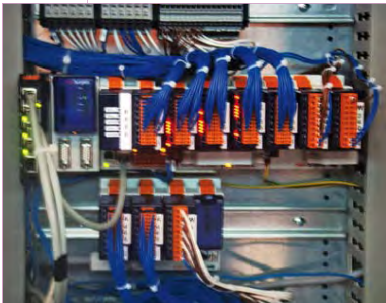
Pumping station control cabinet with Saia®PCD3 controllers
