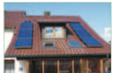
Solar installation on a detached house
