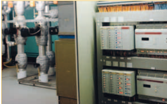
An old system at AMC with Saia®PCD4 systems
