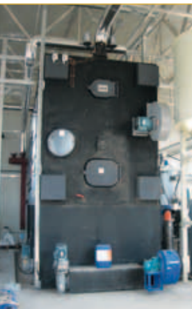
Central heating plant in the Ukraine
