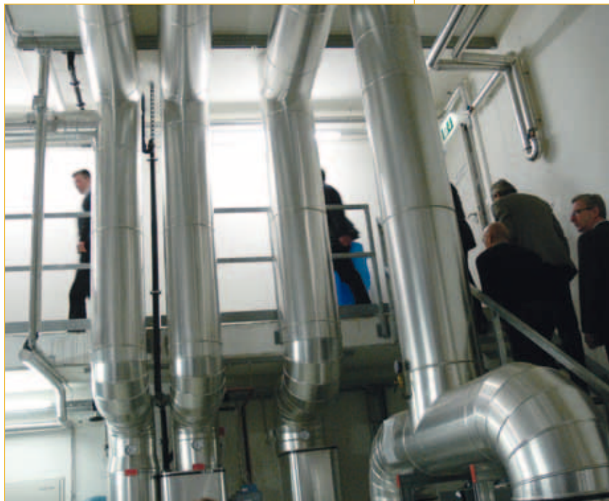
A site visit to an installation was an impressive experience for all customers and interested parties at our events.
