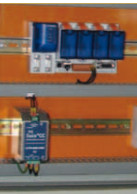
Solar island is controlled with Saia®PCD
