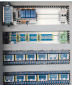
42 Saia® S-Bus energy meters and Saia®PCD3.M3120 controller for energy capture in the airport data centre
