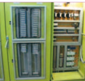
Overall view of switch cabinet including existing Landis+Gyr data point modules
