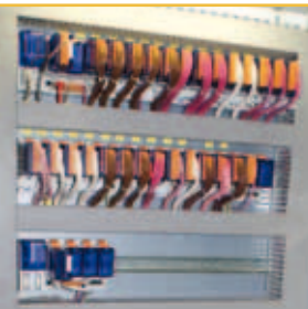
In the new Airport Plaza shopping centre at Hannover-Langenhagen Airport, all building management plant groups are controlled by BACnet®-compatible automation stations of the Saia®PCD3 type
