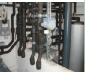
The ATMOVA system from Swissmetal ex- tracts heat from bronze roof tiles. The installa- tion is controlled with Saia®PCD technology
