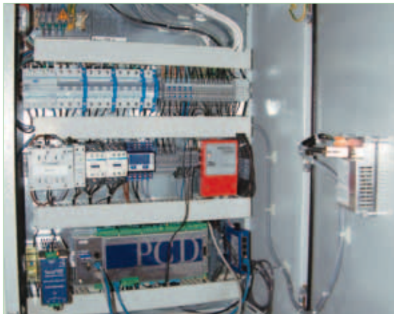
Standardized ATMOVA switch cabinet equipped with a Saia®PCD3.M90 controller (OEM product), a Saia®Energy meter, Saia®Switch, Saia®Supply unit and Saia®HMI
