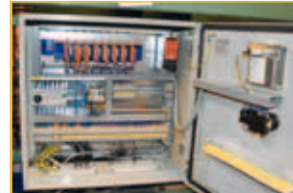
Switch cabinet with Saia®PCD3 controller and PCD7.D232 panel
