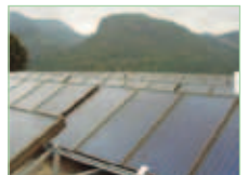
Industrial solar installation
