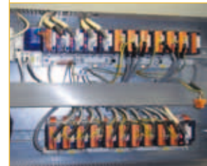
Saia®PCD3 installation in the post and freight terminal
