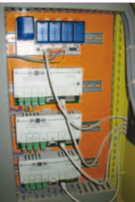
Activation of gateways via Saia®PCD3-CPU
