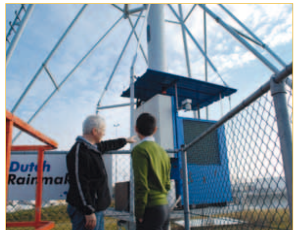
Compressor and switch cabinet directly at the foot of the windmill
