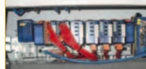
One of the Saia®PCD3 controllers in the premises of Infocontrol Lda
