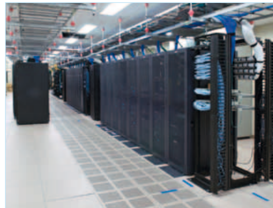
Data centre of Hanover Airport in Germany
