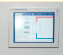
Local operation via a 10" Saia®PCD Micro-Browser Web-Panel on the switch cabinet
