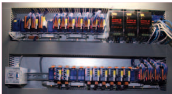
Four controllers from the PCD3 series control the entire heating, ventilation and lighting
