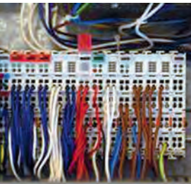
▲ Front image: Tangle of cables in a slice-type control system. Horribly complex and error-prone when it comes to servicing.
