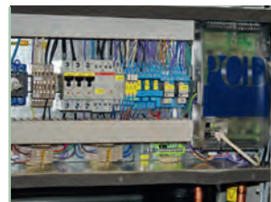
▲ View of ventilation tower control panel with PCD1
