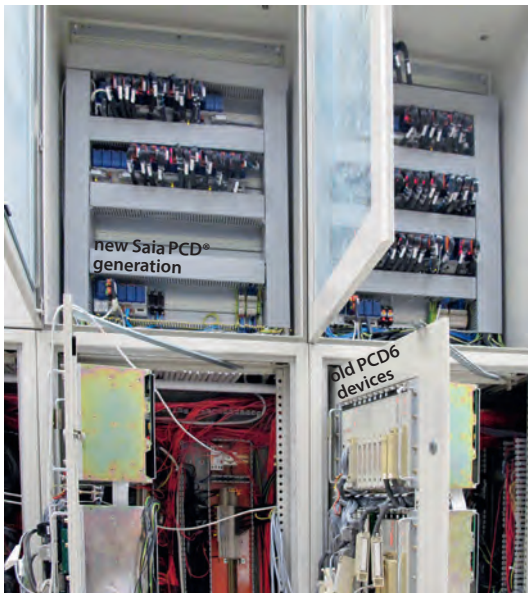
▲ Pictures of the new (top) and old (bottom) panel: The new panel was fitted with PCD3 and tested without stopping production using the "old" PCD6 devices.
