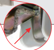
The Achilles' heel of the system: the ground connection of individual bus terminals on slice.
