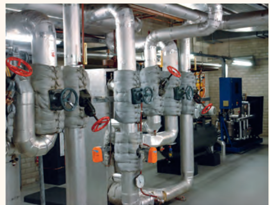
▲ The AMC building The AMC building automation system offers many functions, including peak shaving for electricity and gas consumption.
