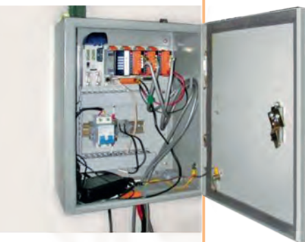
▲ PCD3 to record meter values – everything is not always installed entirely in line with standards
