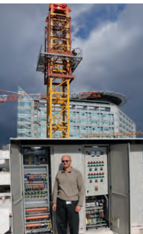
▲ The control panel is located on the roof of the hospital under the fierce sun rays of the Middle East: that posed a challenge for the PLC technology!
