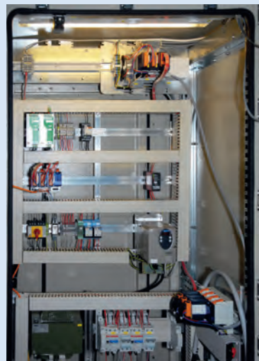
Switching cabinet after the changeover work
