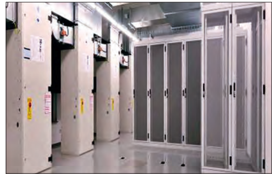
▲ Server room in the Wusys data processing centre Over 500 energy meters and controllers without a control system
