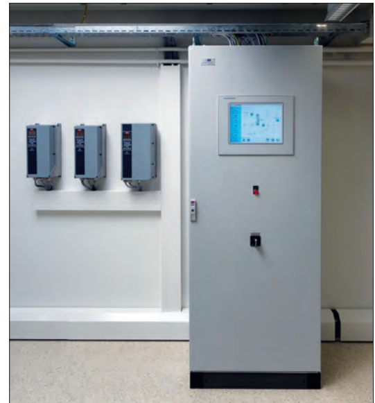
▲ Control panel for the training ventilation facility (Certified POM Gold)
