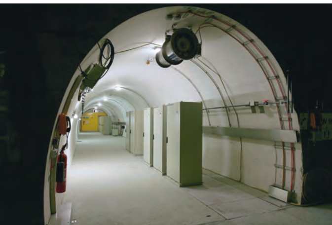
▲ One of 104 cross tubes. Up to 15 switching cabinets can be found in each cross tube.
