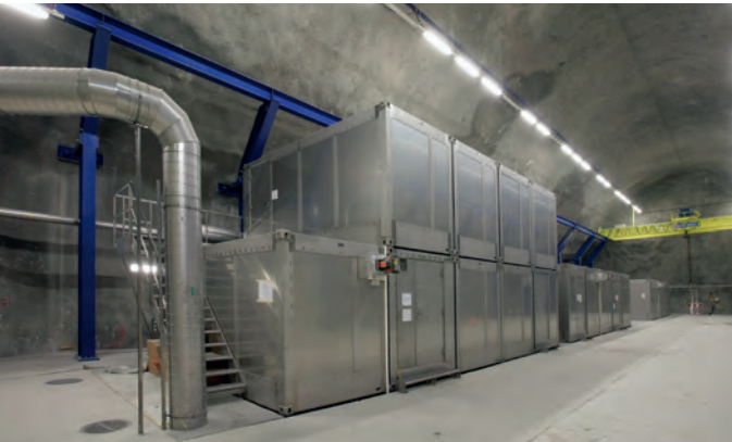
▲ One of 8 tunnel caverns. The railway technology is housed in the air-conditioned stainless steel containers.
