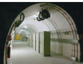
▲ Case study automation/control technology: 34 km Lötschberg Tunnel
