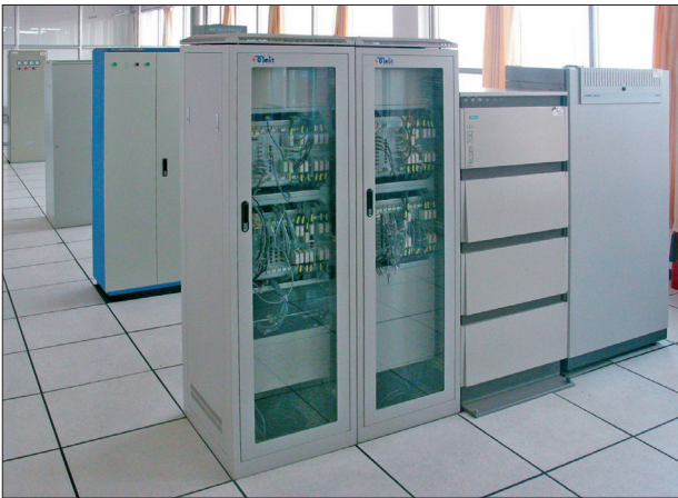
Energy distribution and consumption in billing centre Individual billing of power consumption for shared business premises in offices or industry.
